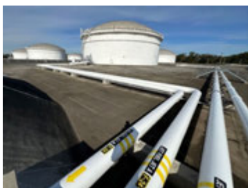
Integrated aviation fuel storage, transfer and hydrant distribution infrastructure supporting modern airport operations
